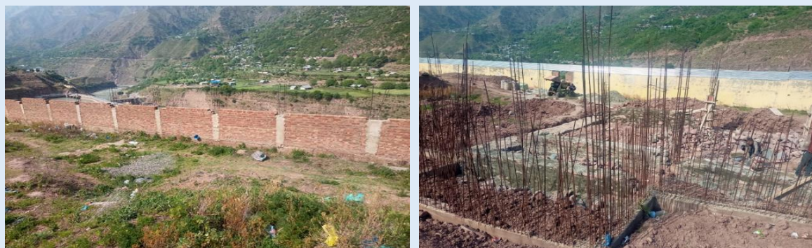
Picture 4.1: Component executed on the land belonging to NHPC at Salamabaad-Uri, J&K, hence the work was stopped and boundary wall was constructed by NHPC
